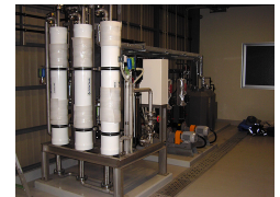
Reverse osmosis membrane unit
