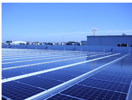
Solar power equipment installed at the Goka Plant
