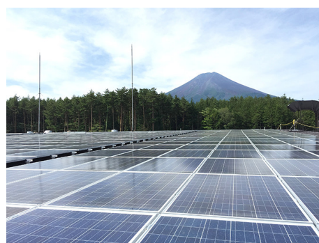
The solar panels of Fujiyoshida Kewpie Co., Ltd.
