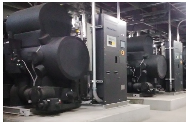
Ammonia freezer units
