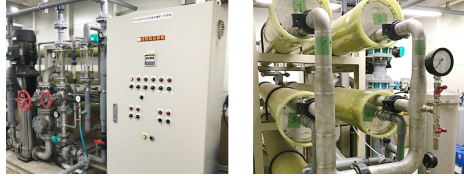
Reverse Osmosis (RO) Filtration Equipment
